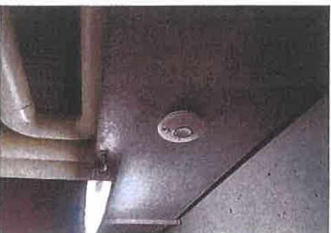
Foto 18: Hercontrole 19/02/2025 - Rookmelder kelder
