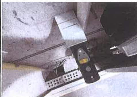
Foto 15: Hercontrole 19/02/2025 - Aarding verdiepingen
